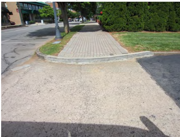
No Ramp Present: not ADA-Compliant
