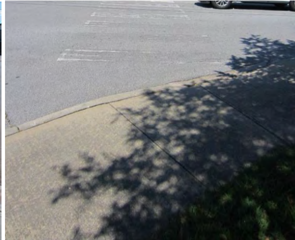
Ramp Present but without Detectable Domes
